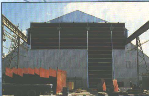
A unique 84' x 55' door with four separate leaves and pivoting mullions at the shot blast shop of Chicago Bridge and Iron Company, Birmingham, Alabama.
